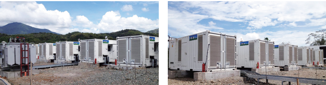
Philippines DMCI group , 18 units APD1513M-6 containerized gensets and parallel operation.
