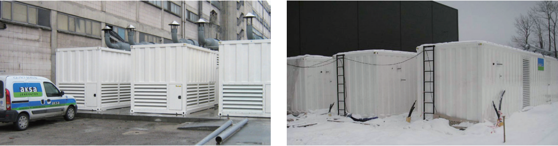
Moscow Ruihao PVC factory , 3 units 2250KVA, 400V container rites gensets runs weaver.
